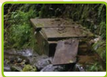
Water collection chamber
